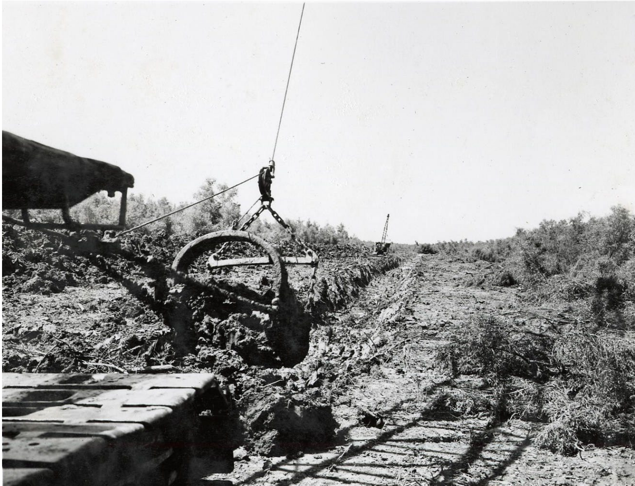
Figure 22.—Looking downstream at excavation of a pilot channel and construction of levee for diversion operations, July 1952 (Reclamation/Herman E. Carter).
